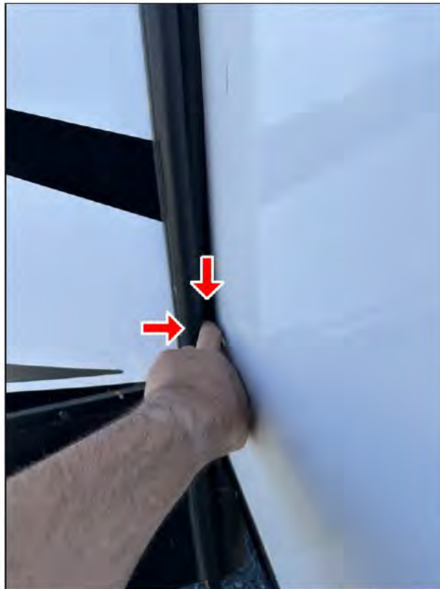
Rear bottom seal of curbside rear slide
