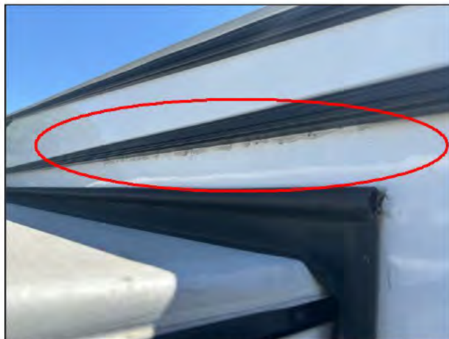
Gutter over streetside rear slide (rear to front)
