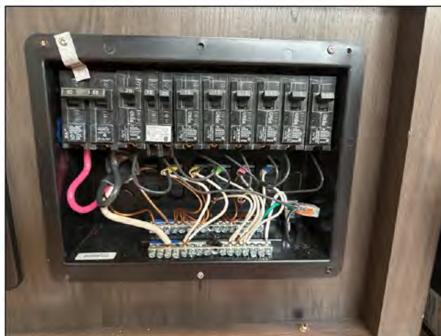
Inside circuit breaker box in bunkhouse below drawers
