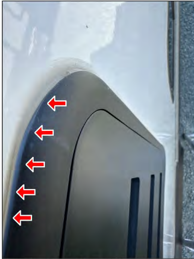
Rear top corner of upper refrigerator vent on streetside
