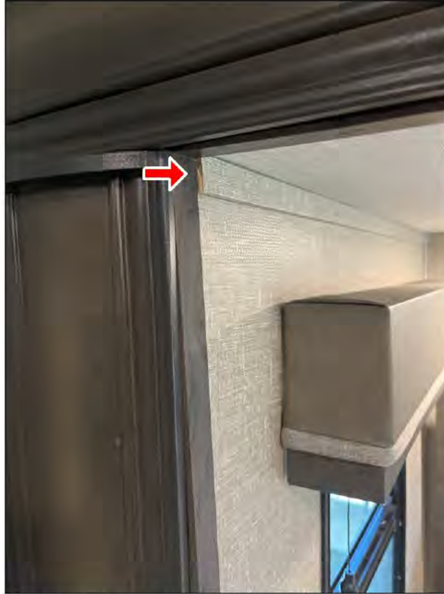
Streetside rear master bedroom slideout ceiling trim
