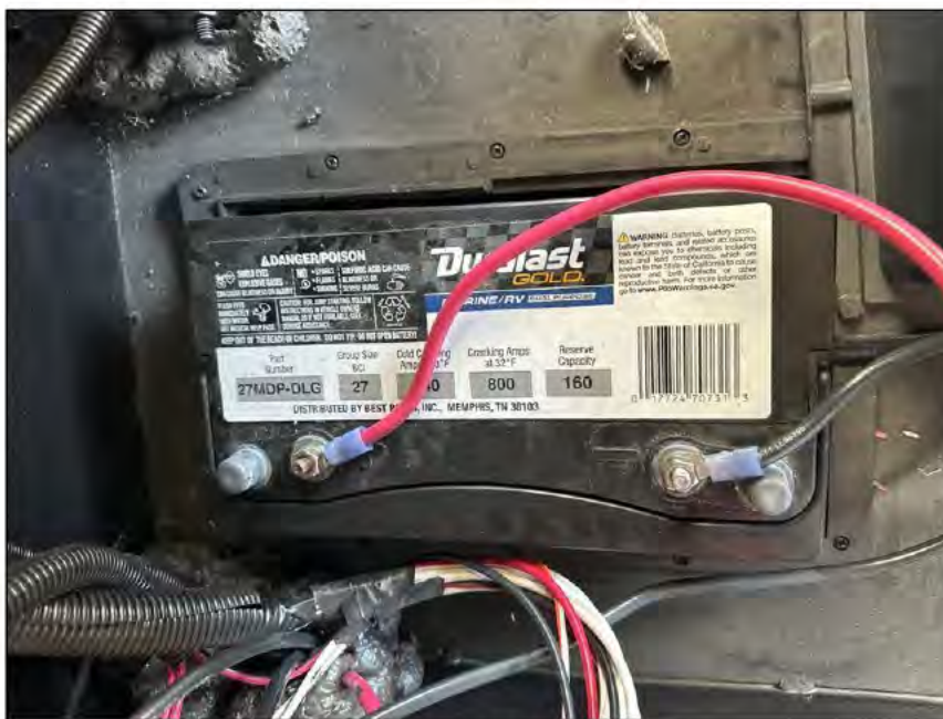
Battery in Front Storage Bay
