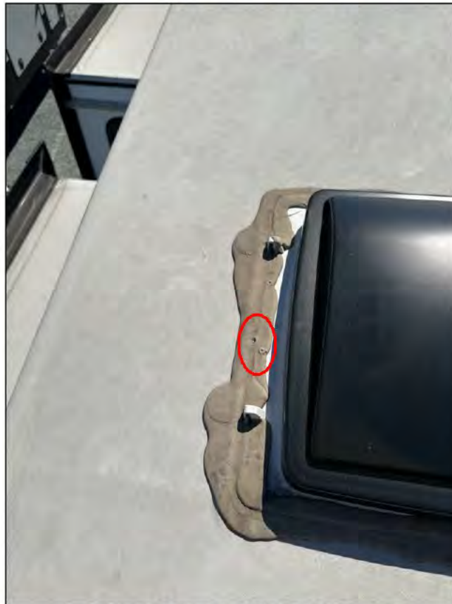
Rear manual vent (from rear streetside)
