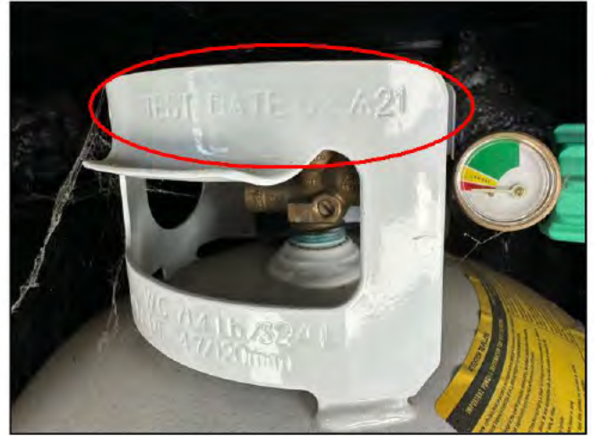
Streetside propane cylinder
