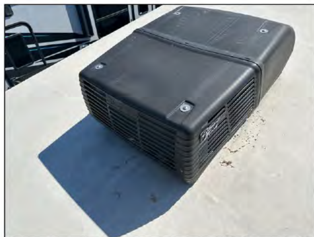
Rear air conditioner cover (rear to front from curbside)
