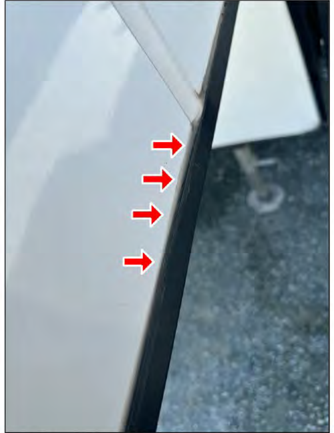
Front streetside side wall from top looking toward rear (closer to front)
