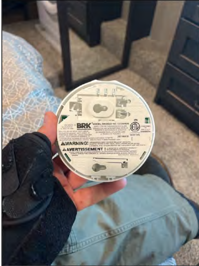
Carbon monoxide detector located in master bedroom
