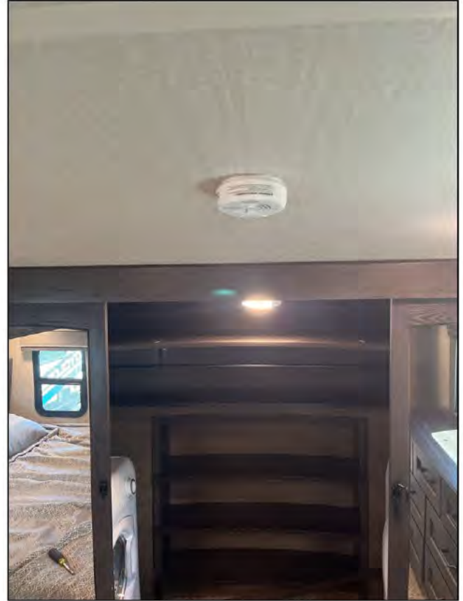
Carbon monoxide detector located in master bedroom
