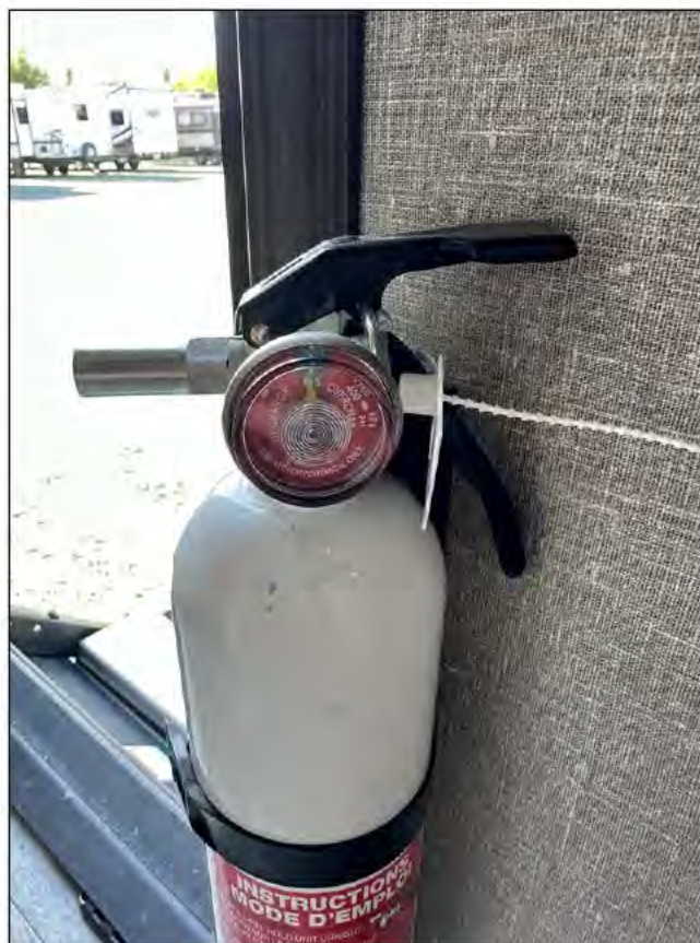
Fire extinguisher inside front door
