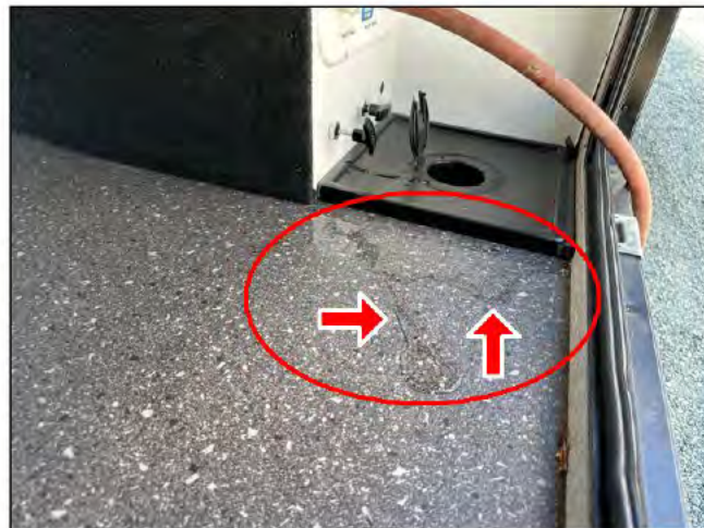
View of Water Control Area in Pass Through (Front to Rear from Streetside)
