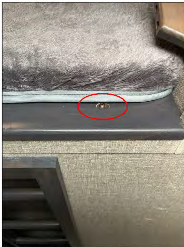
Dented trim on hallway wall that connects to loft
