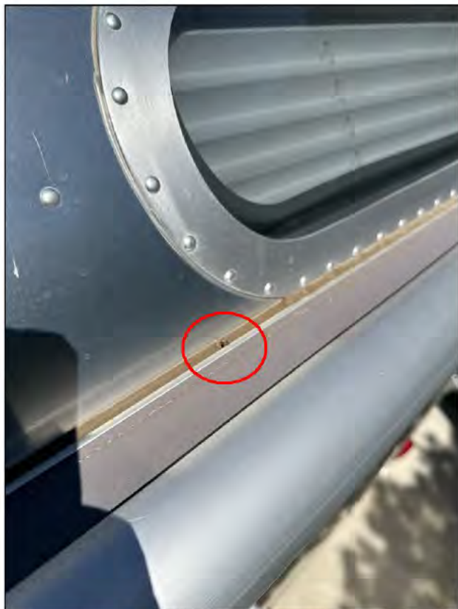
Streetside trim rail over awning under front edge of rear upper window (close up)
