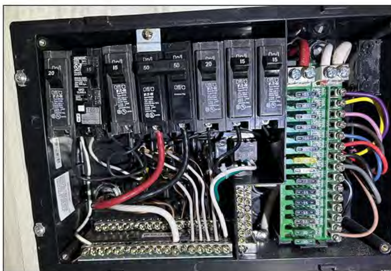
Interior of AC/DC electrical panel under curbside bed
