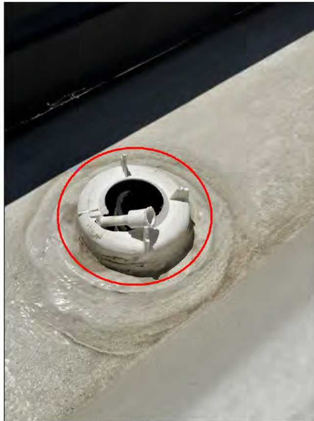
Plumbing vent to the curbside of the bedroom ceiling bump
