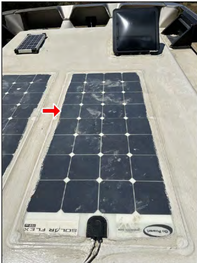
Rear curbside solar panel (100W)
