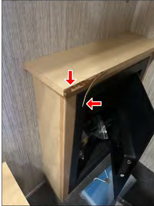
Streetside rear, in master bathroom closet around safe
