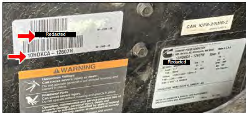
Generator data plate from front cap cargo drawer
