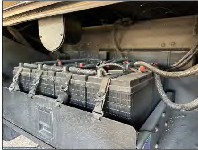
House batteries in streetside cargo bay
