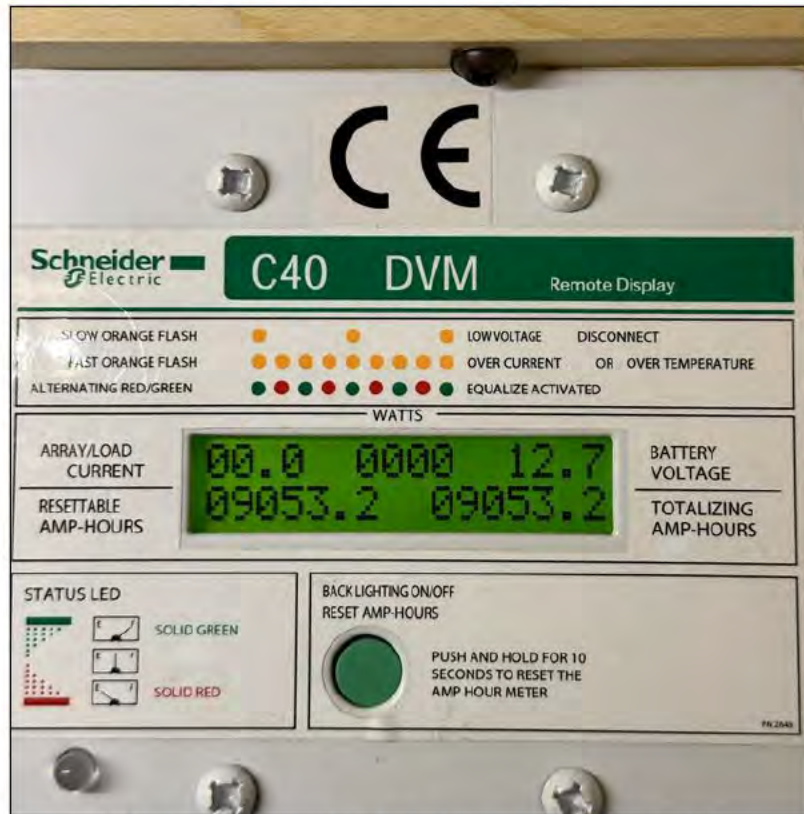
Solar remote display in cabinet over driver seat
