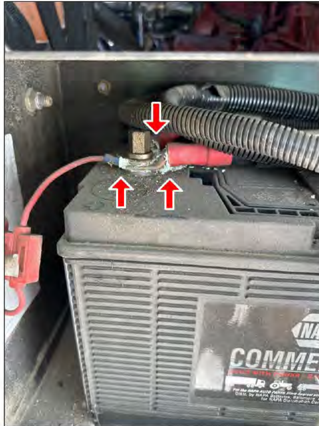
Rear-most chassis battery in curbside rear cargo bay
