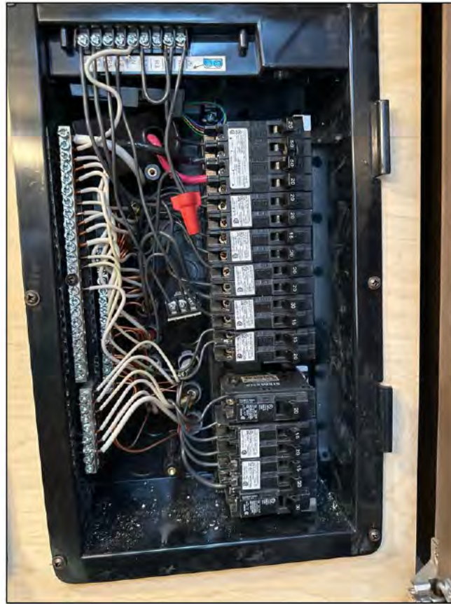
Inside of circuit breaker box in bathroom
