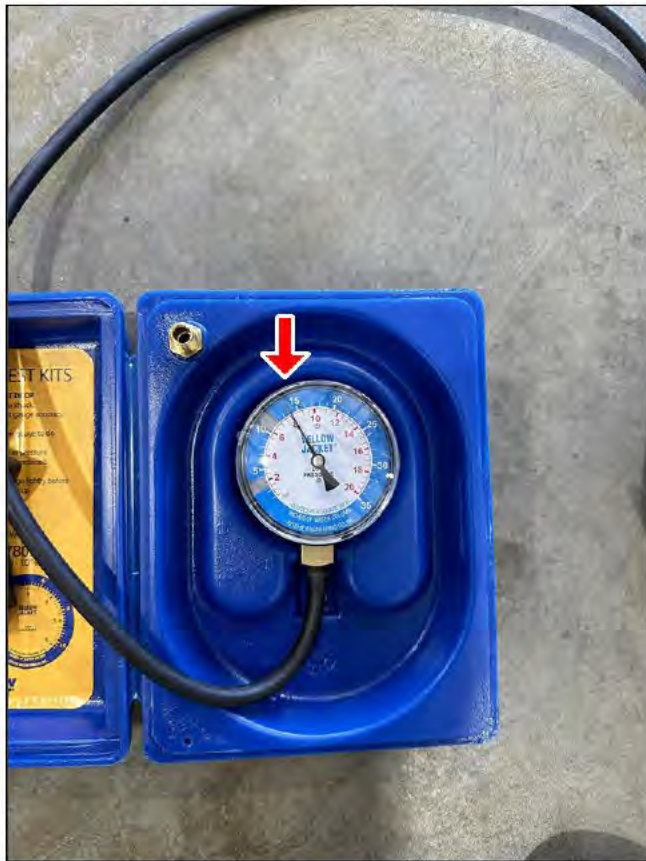
LP pressure gauge showing 14" water column
