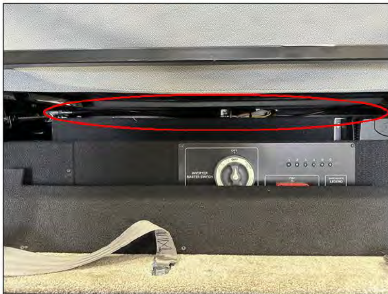
Battery access under the rear couch from rear
