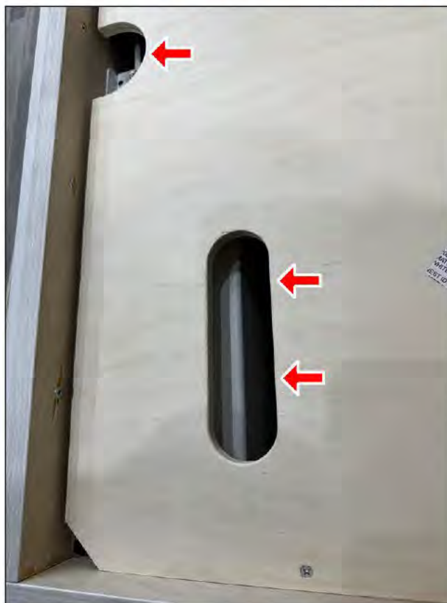
Inverter under curbside rear chair with limited access
