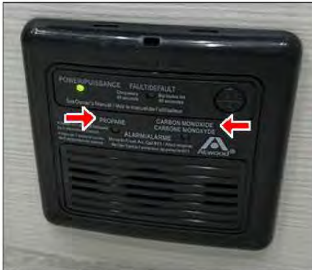
Combo LP/CO detector on streetside under chair (front)
