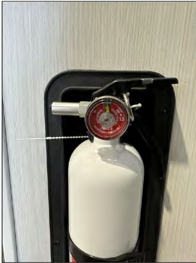
Fire extinguisher inside sliding door (gauge close up)
