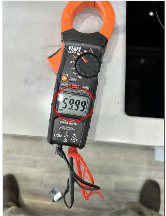
Generator frequency under load at kitchen outlet forward of cooktop
