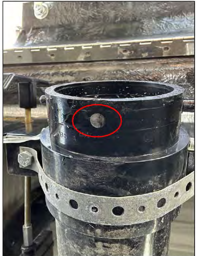
Sewer dump pipe from bottom (from curbside looking up and toward streetside)
