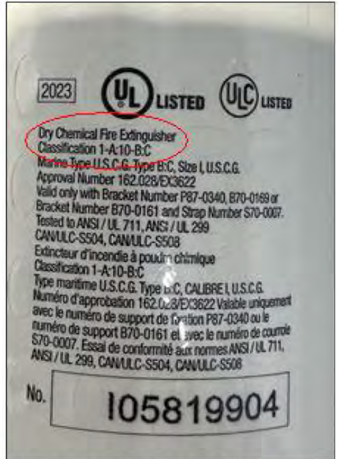
Fire extinguisher inside sliding door (label close up)
