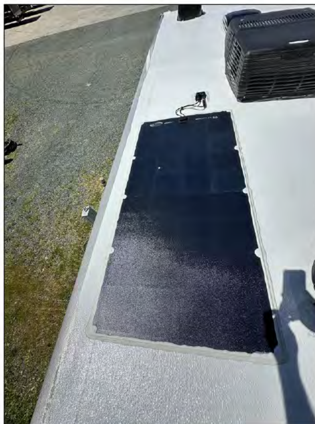
Solar panel on rear streetside (from rear)
