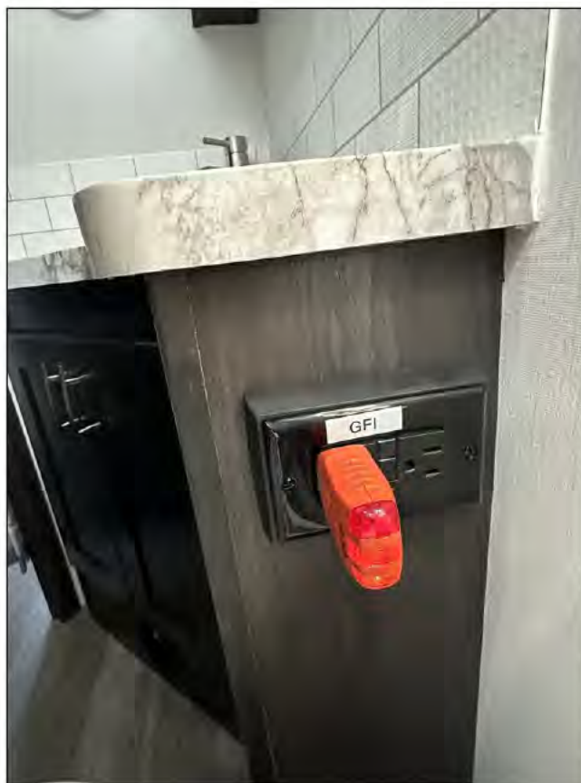
Bathroom outlet next to toilet
