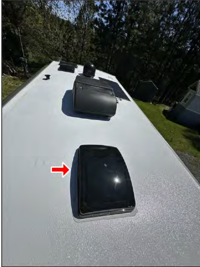
Forward powered vent (from front)
