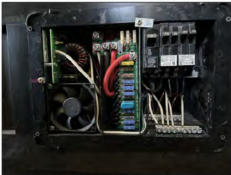
Electrical panel under cooktop
